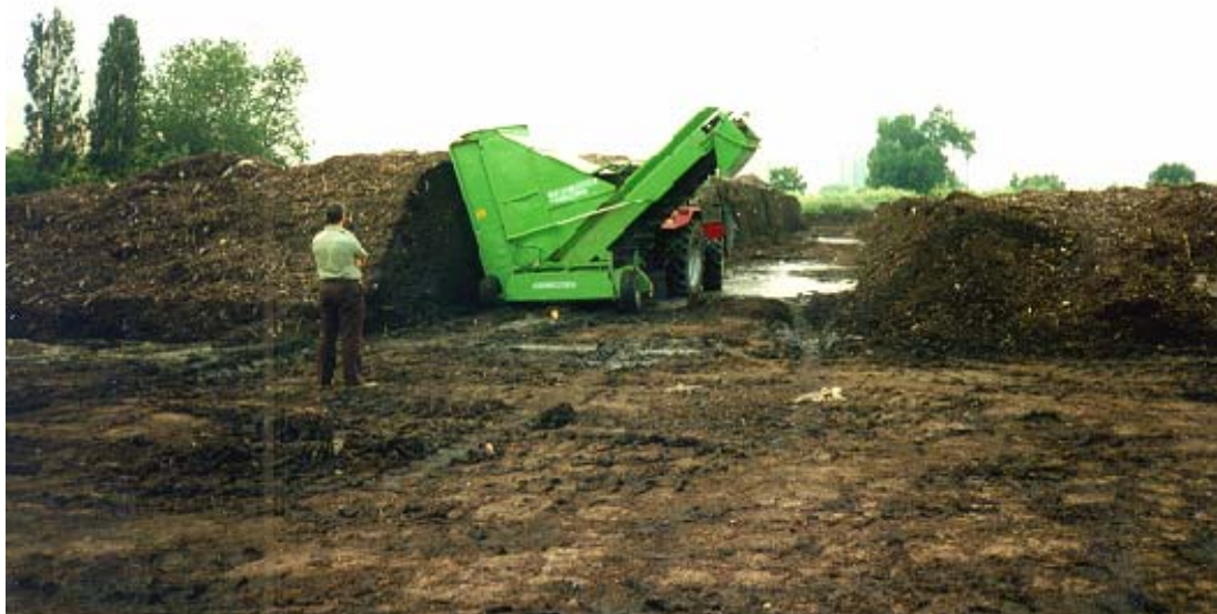
Plate 5.4 Centralised Composting Facility
