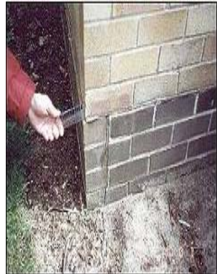
Figure 6.1. Low level sulphate damage to bricks
