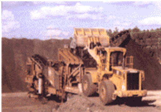
Figure A.4 Loading Of Aggregate Into A Secondary Crusher
